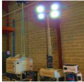
MAIN MOBILE ELECTRICITY SOURCE
